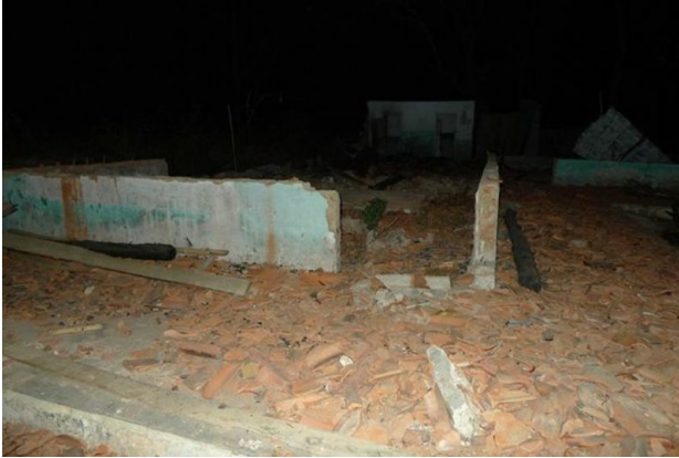
Destroyed Shi'a house at Nanggernang hamlet, Karang Gayam village, Omben, Sampang, Madura
