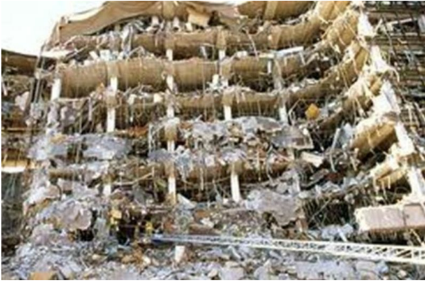
On April 19, 1995, the Alfred P. Murrah Federal Building was bombed, killing 168 and injuring 800.
