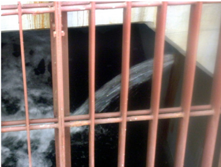
Radioactive water leaks into the sea April 2 from a crack in a pit wall near the water intake of the No. 2 reactor at the Fukushima No. 1 nuclear power plant. (TEPCO)
