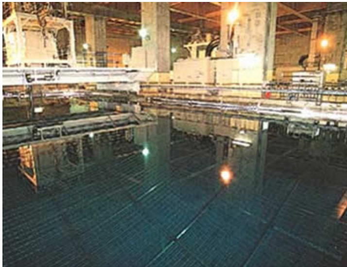
Rokkasho spent fuel receiving storage area
