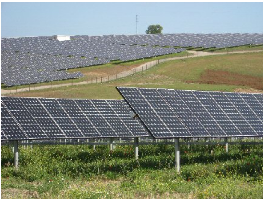
A solar power generation facility
