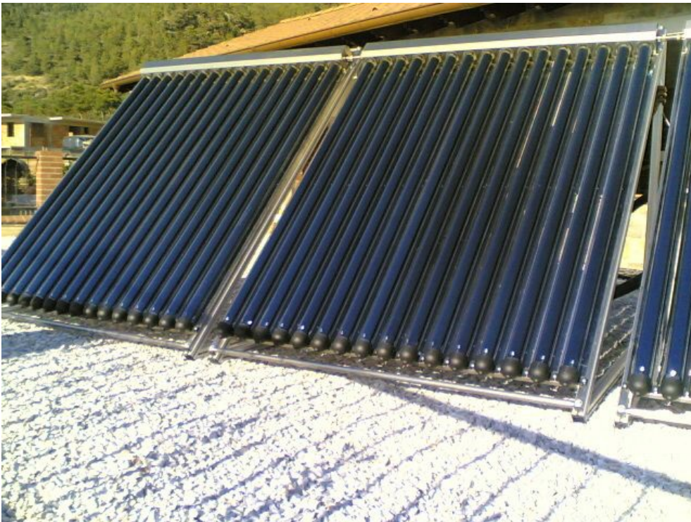
Solar thermal collector, China
