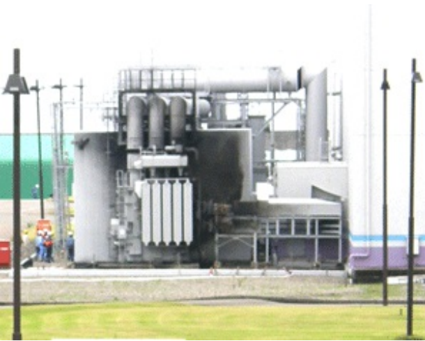
Burnt out transformer at the plant
