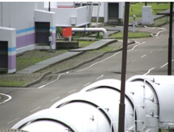
Buckled road at plant site
