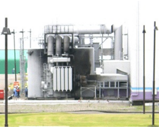
Burnt out transformer at the plant
